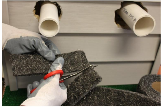
Xcluder brand Fill Fabric getting prepped to fill around a pipe chase.
